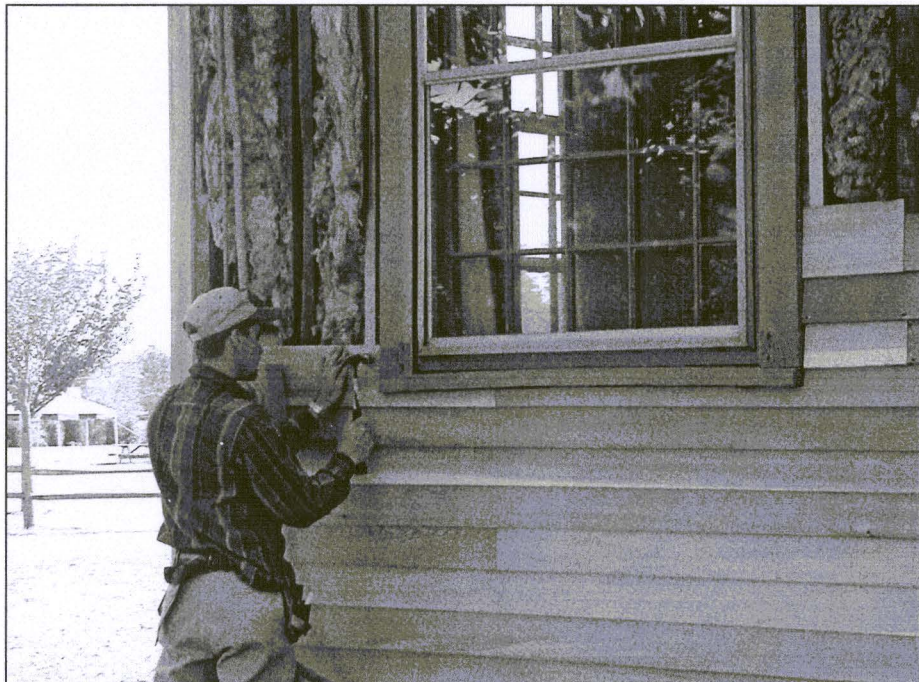
Figure 21. Although the new clapboard was slightly wider than the original, every attempt was made to align the new material with the old.
