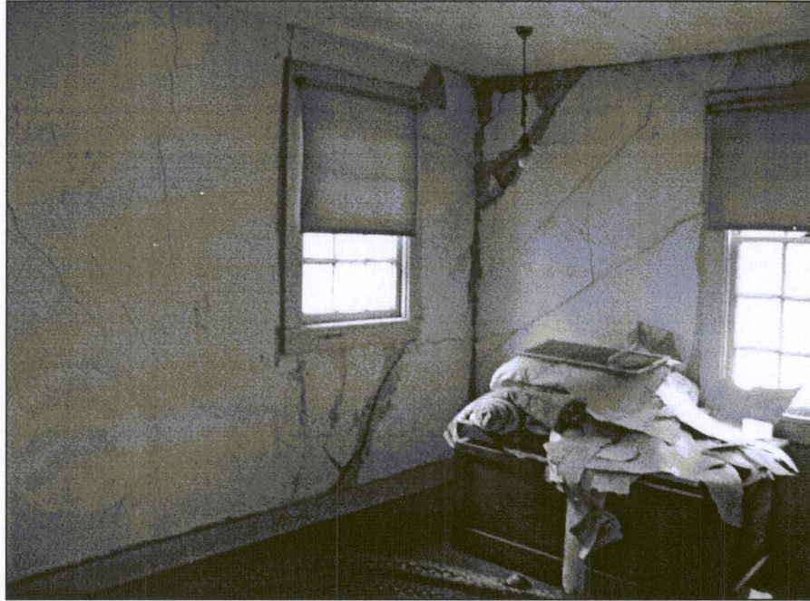
Figure 42. Period 4, second floor (rear room). This room displays the most evidence of structural stress. Measurements of these wall fractures indicate that building's foundation may be settling.
