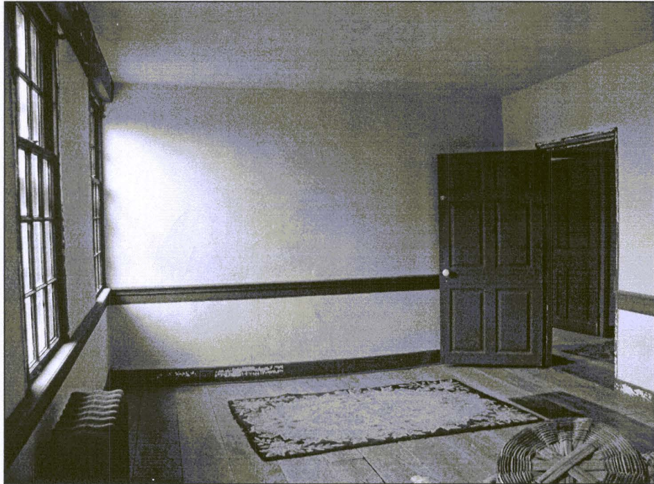
Figure 34. This room is believed to be part of the original Period 1 construction. Located on the second floor, this partition wall divides the Period 1 space, but does not line up with other walls below. Therefore, this wall is considered a “floating wall,” as it relies only on the floor joists and one plate for support.
