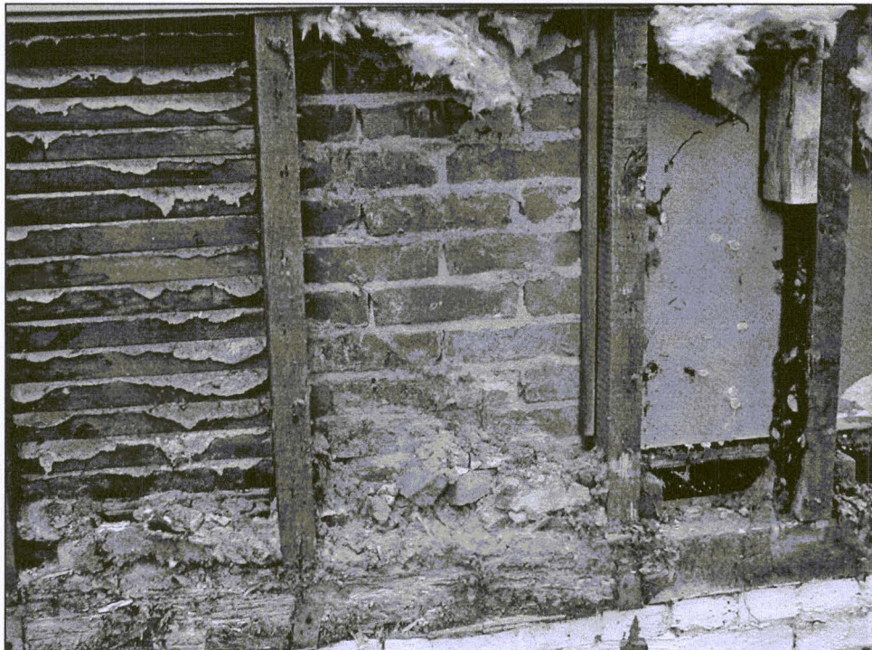
Figure 15. Several wall materials were exposed during the rehabilitation, summer 2000: (R to L) lath, brick chimney stack, and dry wall supported by studs and a deteriorated sill plate.
