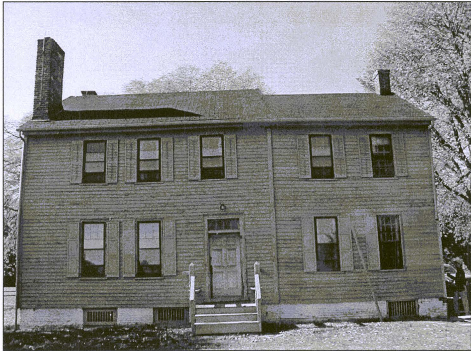
Figure 22. The replaced clapboard is visible along the right edge of the façade above.
