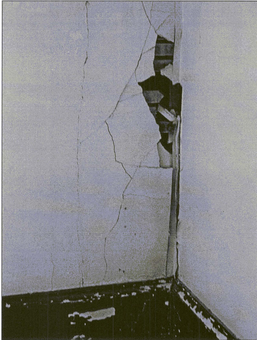
Figure 40. The east corner of Period 4, second floor, (front room) shows signs of structural stress. This detail is found in the rear right-hand corner of the room photographed above. The lath and plaster have pulled away from the corner post.
