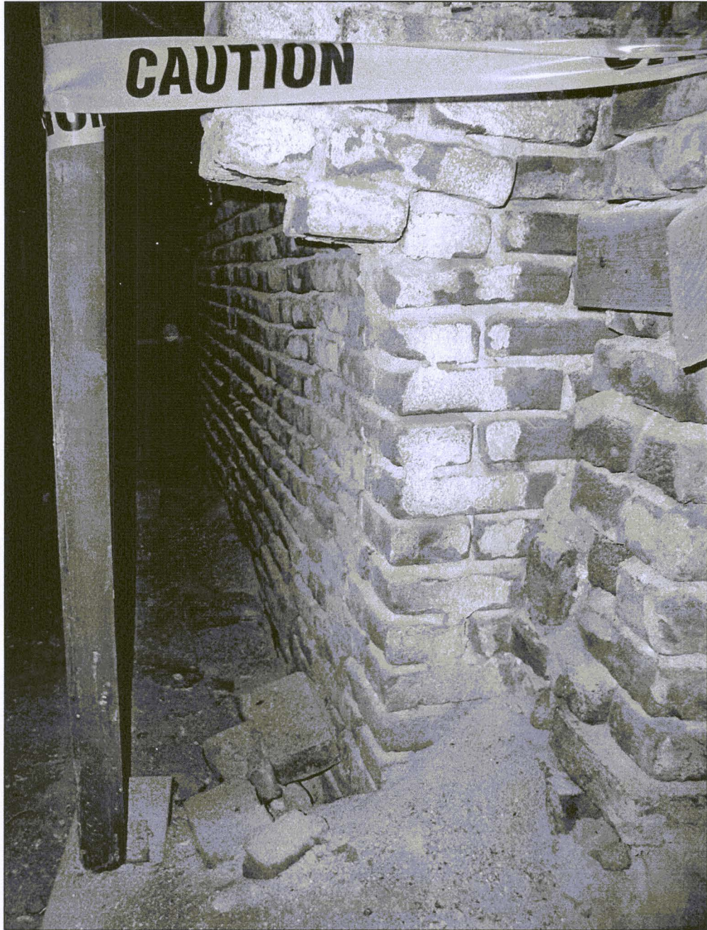
Figure 46. This curious cantilevered wall section in the basement appears next to an abutting wall, mortar dust, and fallen brick.
