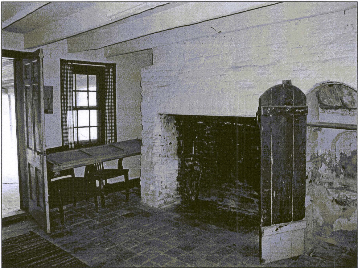
Figure 27. Period 3, first floor, west corner. Note hearth, exposed ceiling joists, and closet containing stove flue.
