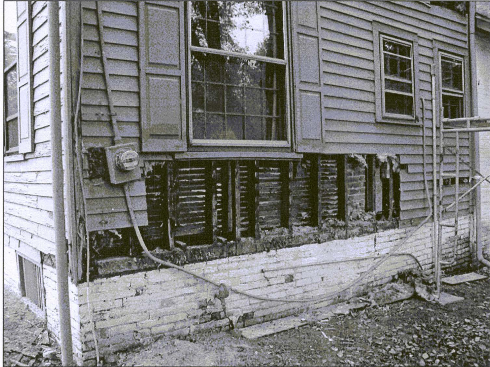
Figure 14. Rehabilitation work on the house during summer 2000 included the partial replacement of clapboard to the Period 4 southeastern and northeastern façades.
