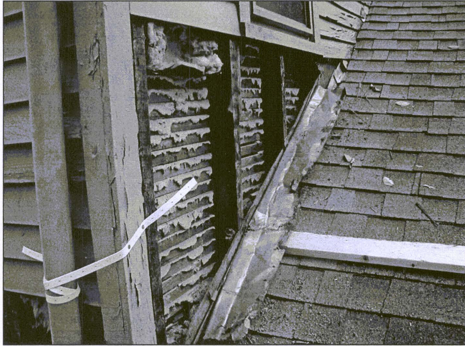
Figure 18. The corner post in the foreground marks the area of most concern. The interior wall of this room is severely marred by stress cracks and fissures in the plaster, indications that this corner of the building is settling. Efforts were made in 2000 to investigate the cause of the structural stress.
